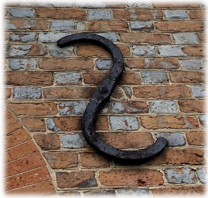
An anchor plate used for structural reinforcement, as seen on the King William Courthouse Square. Many anchor plates are made in a style that is decorative.
